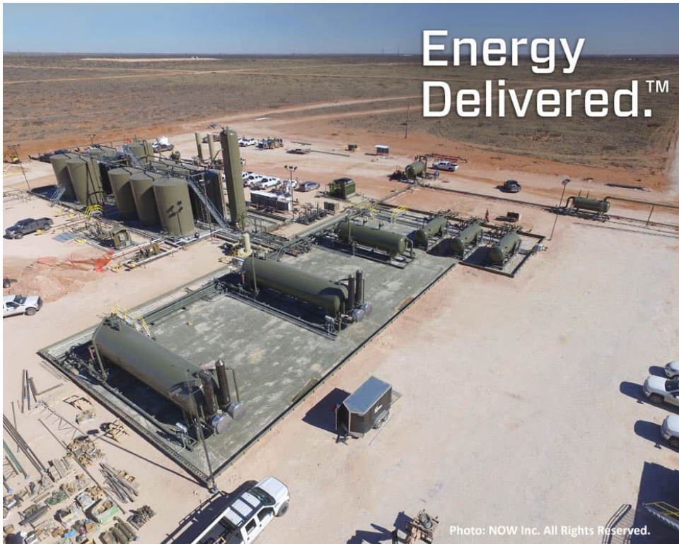
Turnkey tank battery supplied by DNOW
